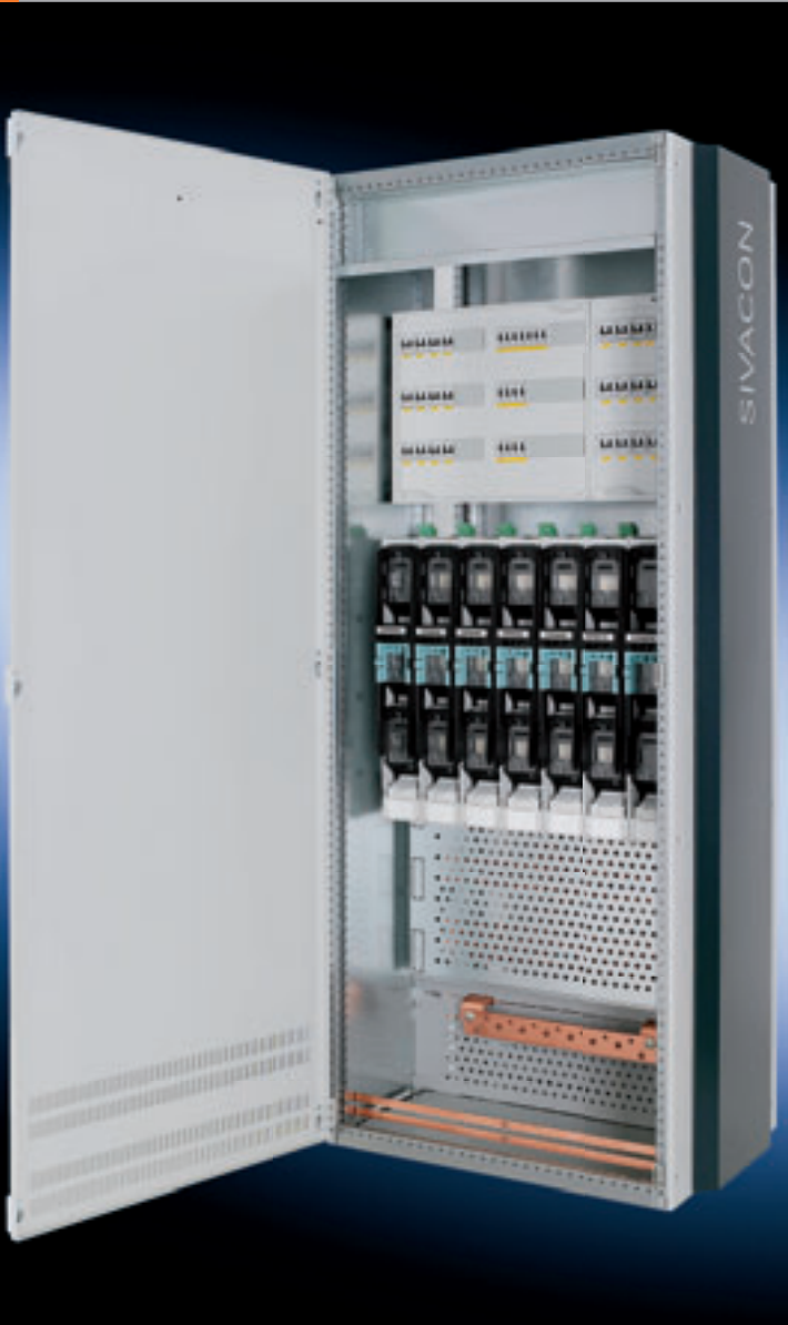
In-line cubicle with 3NJ4 in-line fuse switch disconnectors and rapid mounting kits for built-in installation devices
