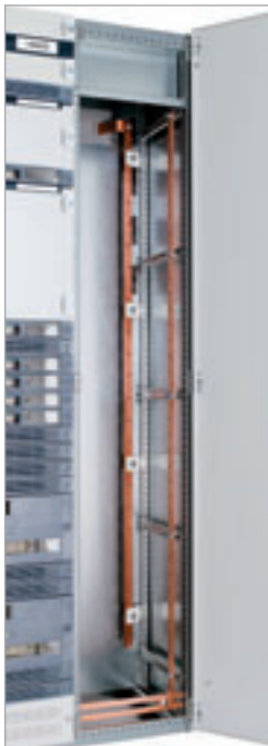
Vertical PE and N conductor rails arranged in the cable connection compartment at the right
