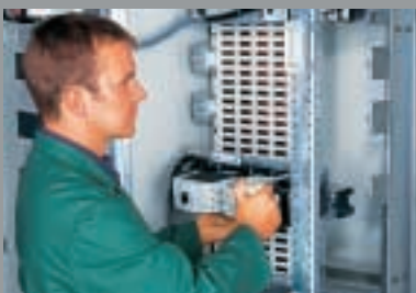
Plug-on bus system Guide rails (short and long) on the left- and right-hand sides of the cubicle
